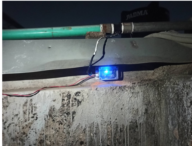
Water flow monitoring unit
